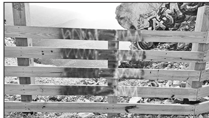
One example of the vandalism that has occurred.
